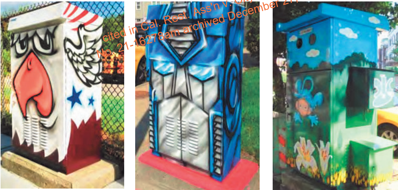
Figure 1 Examples of Enclosures in Violation of Note 2 (above)
